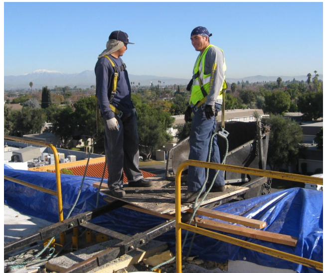
Workers from Honeycutt are properly secured with fall protection while working on the roof.
